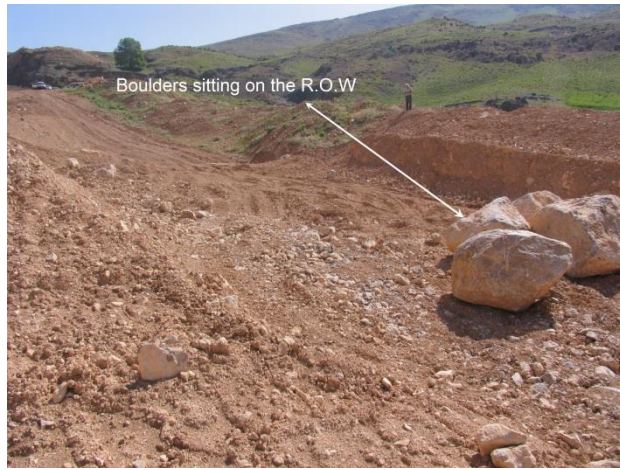
Figure 6. Large boulders closing the R.O.W due to the soil movement
