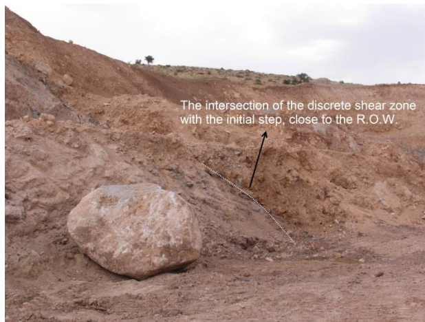
Figure 15. The intersection of the discrete shear zone with the initial step above the R.O.W
