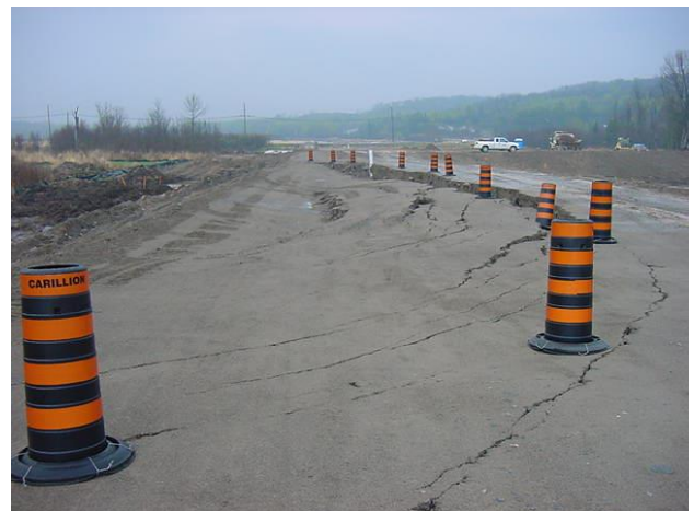
Figure 10 – May 10, 2005 – Embankment Failure
