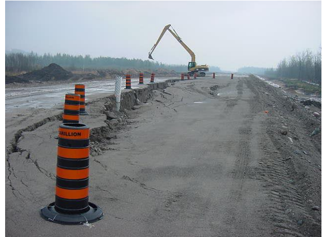
Figure 8 – May 10, 2005 – Embankment Failure
