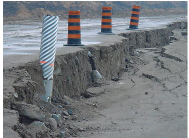
Figure 9 – May 10, 2005 – Embankment Failure
