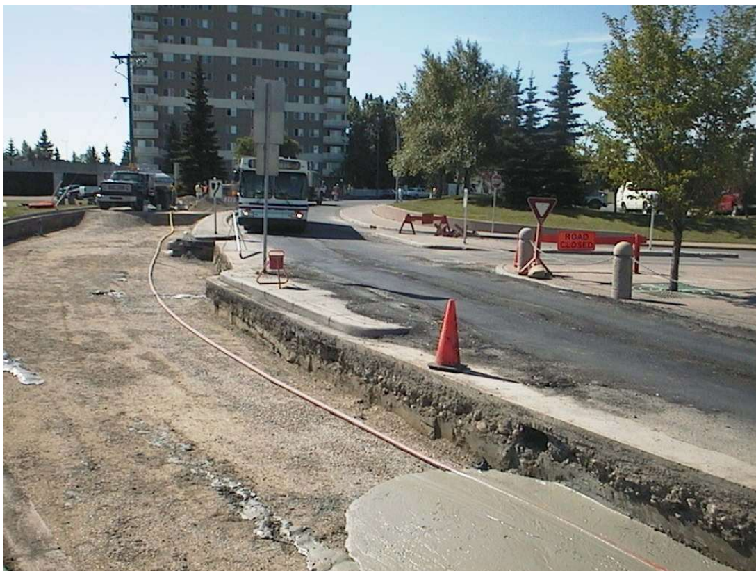
Figure 2. Condition of bus lane (taken during reconstruction)
