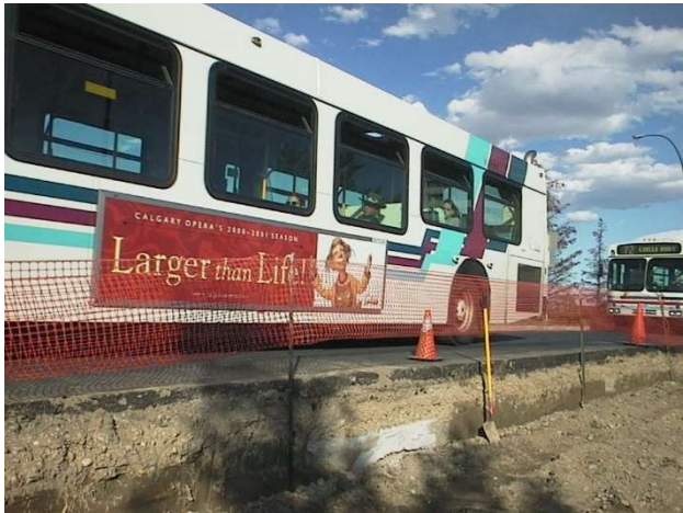
Figure 7. Excavation prior to July 29, 2000 placement of cellular concrete. Note exposed LCC from previous pour.
