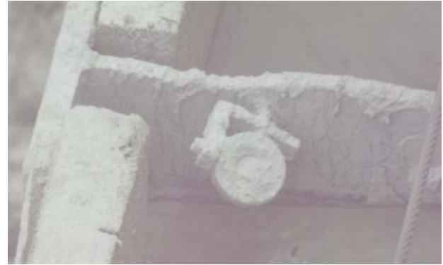
Figure 4. A close-up image taken by an AMTS camera showing a prism covered with grout at the top of a support of excavation.
