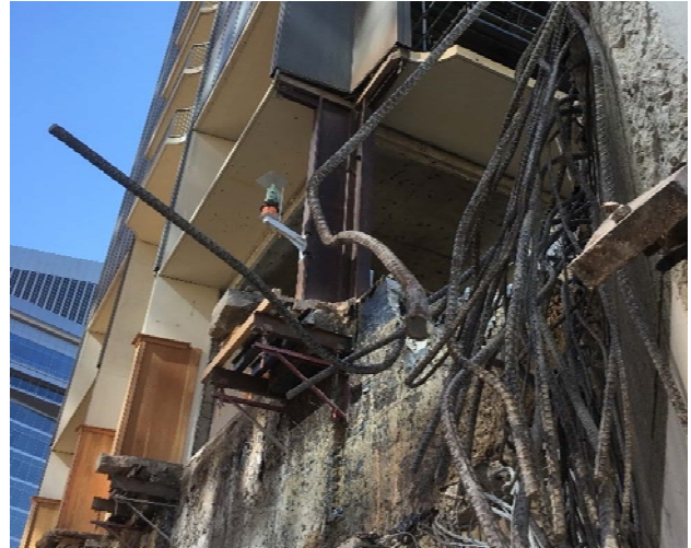
Figure 5. Use of an AMTS to monitor the shoring structures of an urban excavation, as well as adjacent buildings. Confidential project (downtown Los Angeles, CA)
