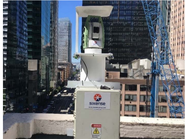
Figure 2. Typical AMTS installation on a roof top. Monitoring of an adjacent urban excavation for vertical construction
