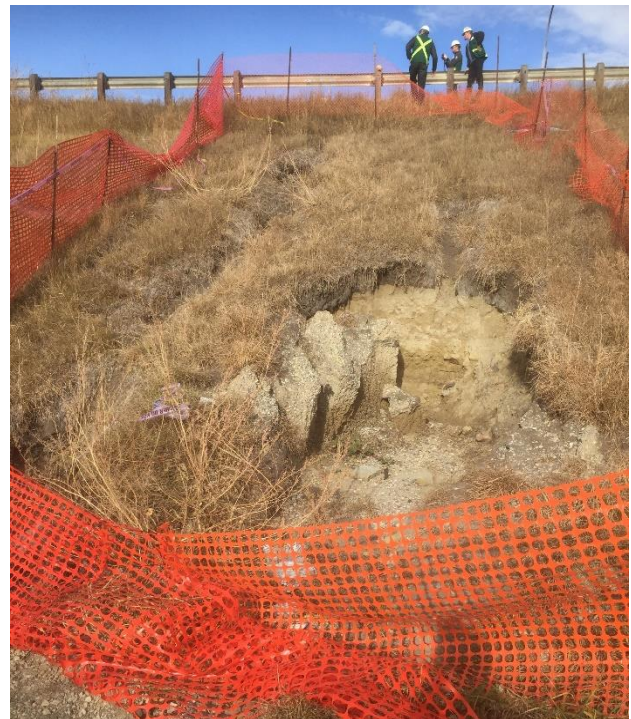
Figure 4. Well-vegetated slope sloughing after thirty years
