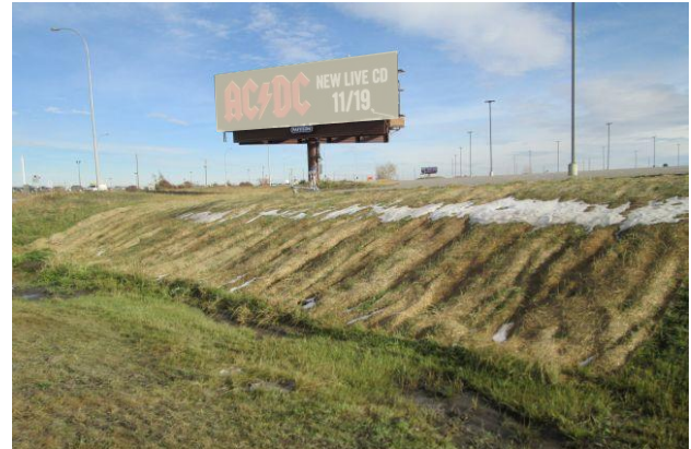
Figure 6. Erosion below Rolled Erosion Control Blankets not conformed to soil surface
