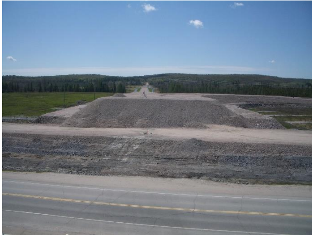
Figure 5 – Looking West at West Approach during Surcharging
