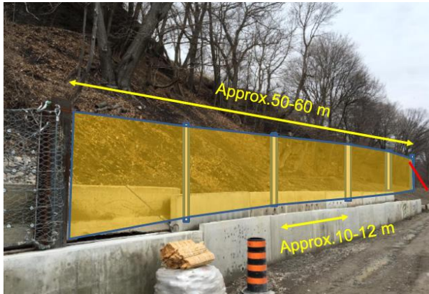
Figure 9. New 500kJ rigid post rockfall extension concept attached to previously installed system viewed upslope
