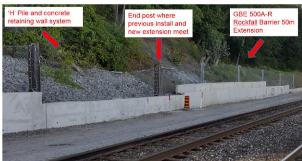
Figure 14. Transition area where the previously installed system is connected to the 50m long new extension
