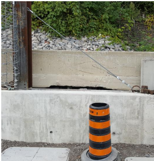
Figure 5. Robust 'H' pile stiffened to prevent buckling during impacts. Additional lateral post ropes also were utilized
