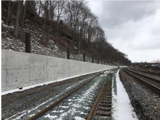
Figure 7. Completed Hybrid 'H' pile and concrete retaining wall view downslope of the barrier
