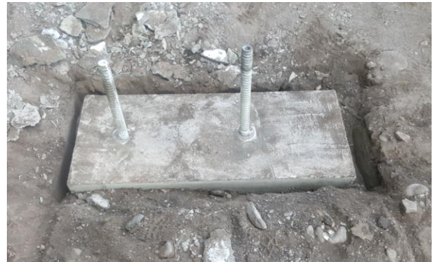
Figure 11. Concrete leveling pad with hollow core anchors visible prior to testing and installing rigid barrier posts
