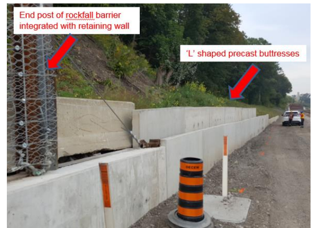
Figure 8. Precast 'L' shaped concrete buttresses used to prevent soil from raveling onto the track expansion
