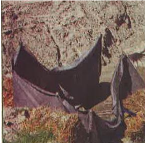
Figure 1. A sinkhole above the TBM
