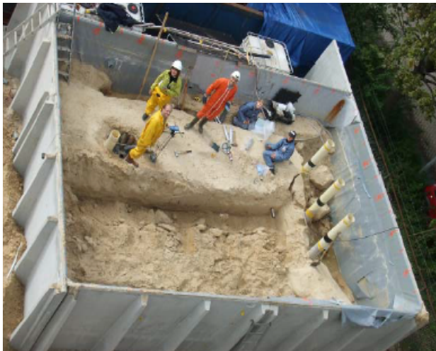
Figure 5. 100 m 3 container provided by VSF company and used by Soletanche-bachy (Esnault-Filet et al. 2015).
