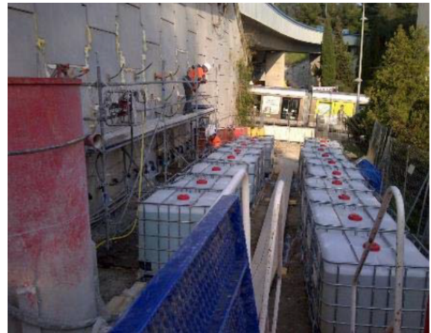
Figure 6. Reinforcement of soil retaining wall using Biocalcis® at field scale (Esnault-Filet et al. 2015).
