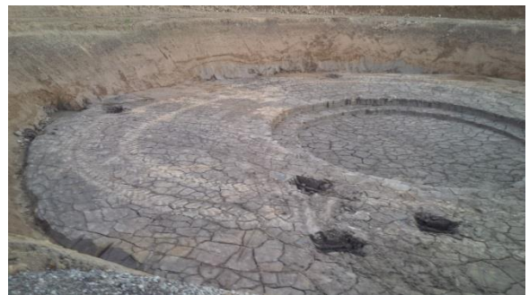
Figure 4- Soft Clay subgrade, showing desiccation cracking.
