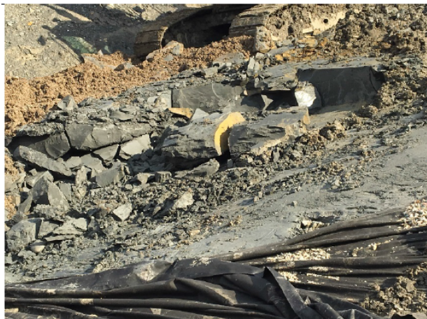
Figure 9. Removal of disturbed and pre-sheared bedrock down to competent bedrock using a tracked excavator.
