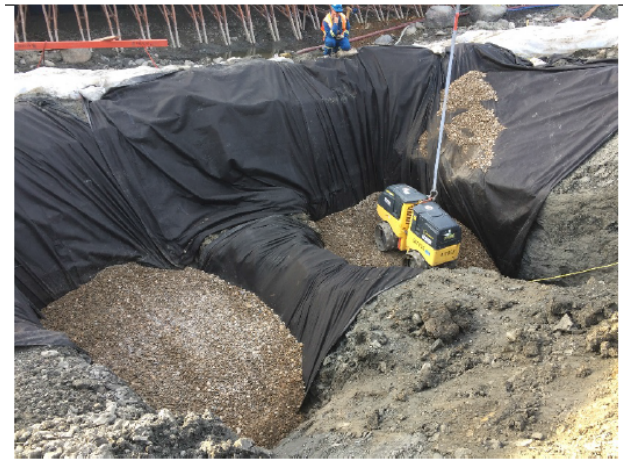
Figure 10. Remote control compactor compacting granular backfill after removal of soft clay infill in the bedrock anomaly at the river bottom near the toe of the slope
