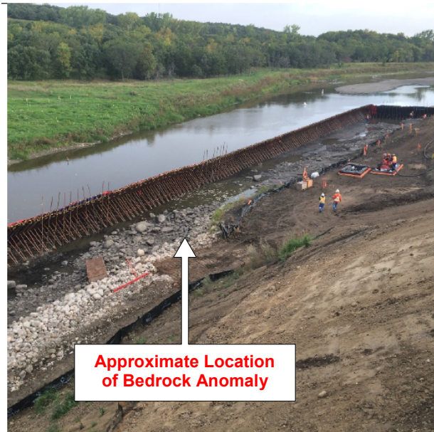
Figure 8. Temporary Portadam structure to allow the remediation to be carried out in the dry.
