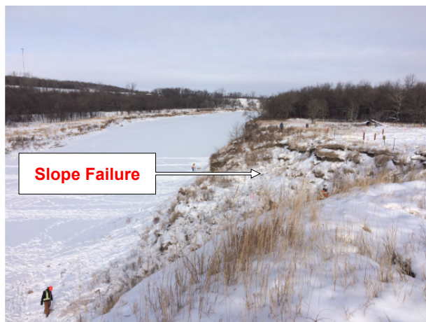
Figure 2. Riverbank slope failure, January 2016 (East bank of Souris River looking north or downstream)
