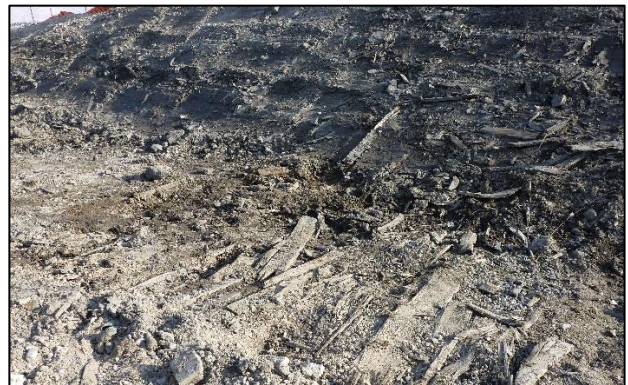
Figure 4. Photo of exposed fill subgrade with wood debris.
