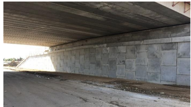
Figure 4 – Actual Photo of North Wall on August 28
