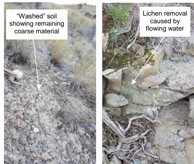
Figure 4. Raveling of fine material and removal of lichen
