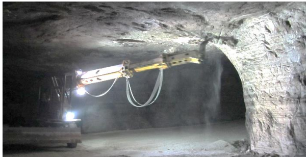
Figure 1.2: Mechanical scaler cleaning the surface of a pillar after a blast at the Ojibway mine (Windsor, Ontario, Canada). The room is approximately 6 meters in height and 13 meters in width.
