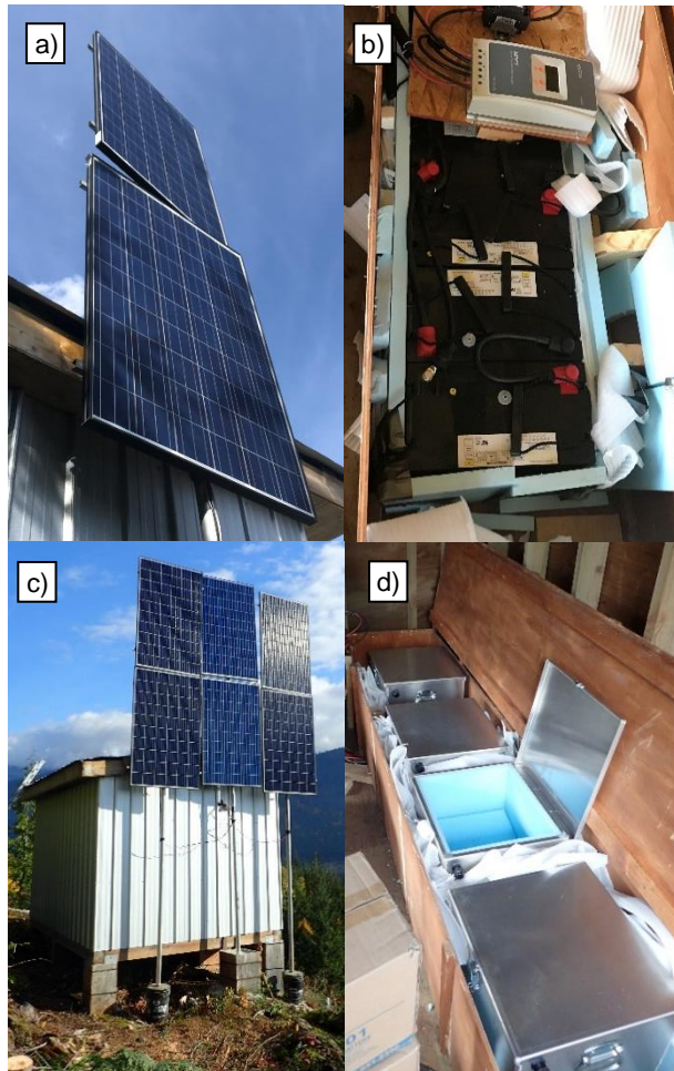
Figure 4: Original solar panel installation Oct 2016 – Oct 2018 (a) and battery pack and 20A charge controller (b). Upgraded solar installation Oct. 2018 – Present (c) and insulated aluminum battery boxes (d)
