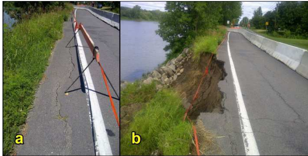
Figure 4. (a) Pre-failure warning sign of a landslide (arc-shaped crack in the shoulder) and (b) landslide, occurring before stabilization work
