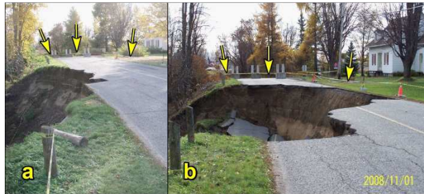
Figure 2. Example of a safety perimeter (closure of the road, indicated by the yellow arrows) having foreseen the spatial evolution of the next land movement to occur: (a) the landslide's initial scar and (b) enlargement of the scar
