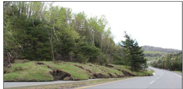
Figure 3. Example of a landslide whose debris spread halfway across the road
