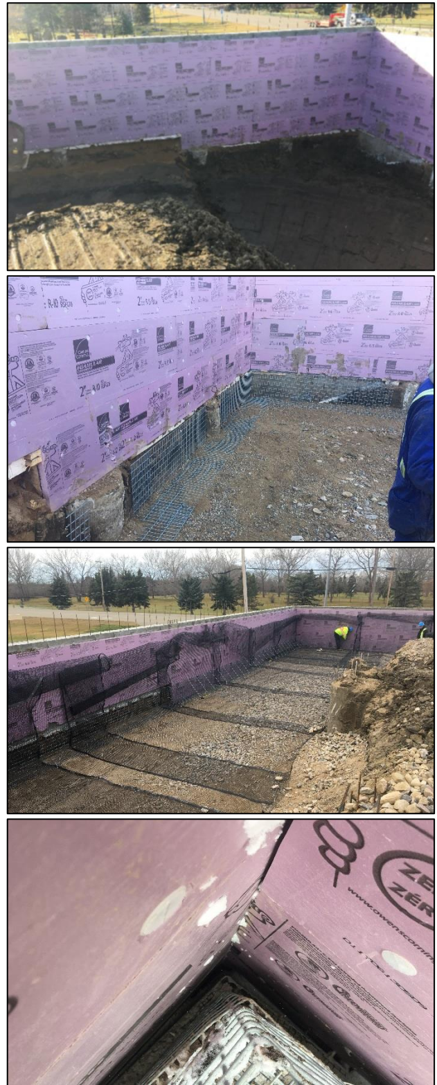
Figure 5. Construction photos of GRE construction, starting from top, showing prepared subgrade, first row of wire-mesh baskets, geogrid installation, and desired gap between grade beam and GRE structure
