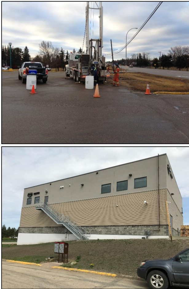
Figure 1. Pre and post construction of the proposed building with grade beam wall ranging from 0.3 m to 3.0 m in height
