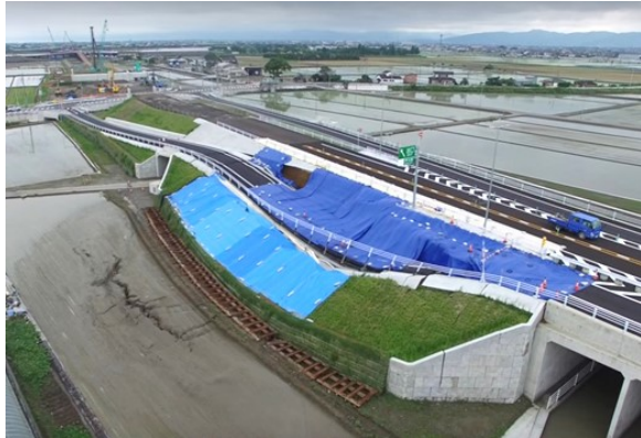
Figure 1. Collapse at Ashikari-minami Interchange (Saga, Japan) (Miura and Hino, 2018)
