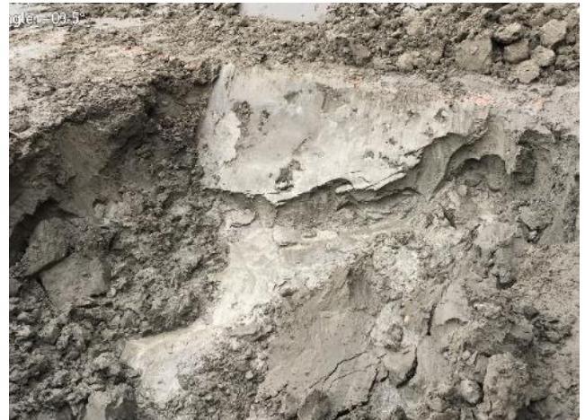
Figure 10. Sloughing soil in Tower Crane 1 test pit
