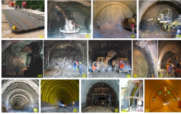
Figure 2. Sequencing of tunnel construction at selected stages; (a) forepoles, (b) installation of forepoles at tunnel face using forepoling machine, (c) view of tunnel face with forepole umbrella inserted, fiberglass dowels, and drainage pipes, (d) shotcrete being applied, (e) controlled excavation of face, (f) excavated material, (g) removal of excavated material, (h) installation of structural support – steel sets, (i) installation of further radial support – grouted rockbolts, (j) successive forepole umbrella seen as well as bench, (k) installation of geomembrane, (l) installation of steel reinforcement for final lining, (m) detail of reinforced final lining, and (n) completed tunnel (Vlachopoulos 2009)
