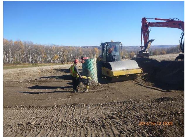
Figure 4. Extending instrumentation (inclinometer and VWP) through the embankment fill using ribbed large diameter plastic conduit and careful hand packing of sand inside the conduit and careful packing of berm fill around the casing exterior.
