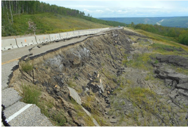
Figure 2. Further retrogressed south slope in July 2015, showing a 6.5 m drop in the pavement.
