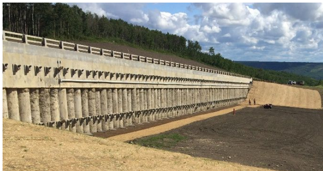
Figure 7. Pile wall completed and south slope of the embankment backfilled to final grade just below the middle row of ground anchors.
