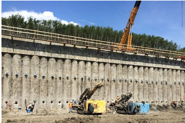
Figure 6. Initial excavation of the area immediately south of the pile wall to a depth of 10.5 m below the pile cap to allow for anchor installation.
