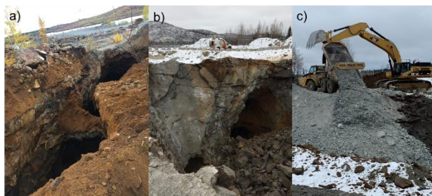
Figure 7: Stope 1-15E a) Initial crevasses b) Opening exposed after blast c) Backfilling
