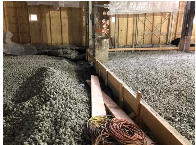
Figure 11. Construction of UL-FGA at the Starrett-Lehigh Building in Manhattan. The area to the right is compacted and ready for slab construction.
