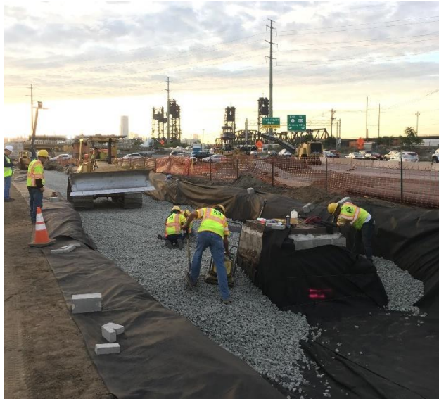
Figure 10. Construction of Route 7 in Kearny, NJ. Note the reduced lift thickness and plate compactor around the inlet.
