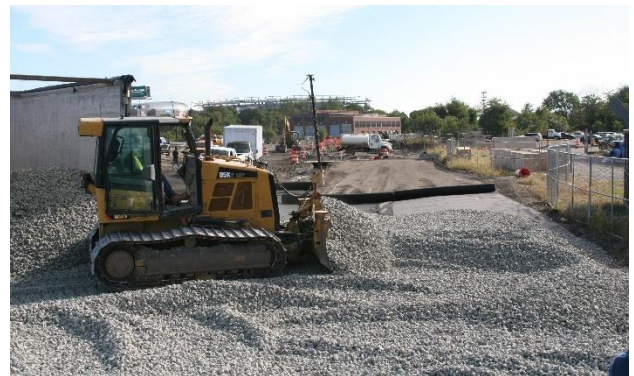
Figure 9. Construction of Langley Avenue in Philadelphia, PA during placement and compaction of UL-FGA
