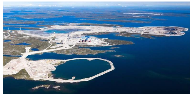
Figure 6. Aerial view of the A21 Dike (foreground) looking north during construction of the COW in 2017. On the right (background), A418 and A154 Dikes and open pits.
