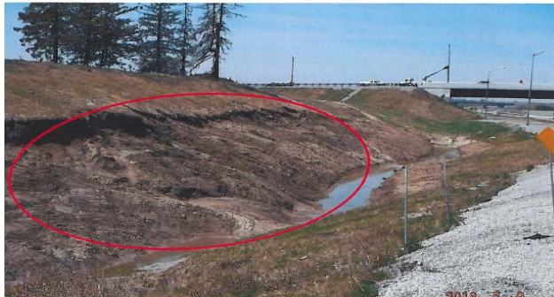
Figure 2. Example of local failure (Ontario 400 Series)
