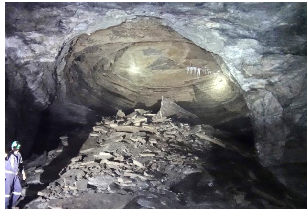
Figure 12: Roof collapse due to time-dependent relaxation
