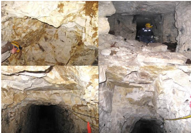
Figure 15: Progressive collapse of roof slabs due to weathering/seepage loss in vertical joints and abutment relaxation (after Diederichs and Hutchinson 2019).
