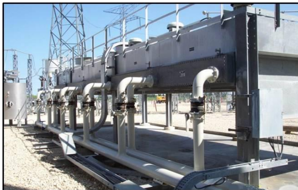
Figure 7. Manitoba Hydro Dorsey AC/DC Converter Station Geothermal System New Glycol Winter Chiller (R. Sinclair 2003).
