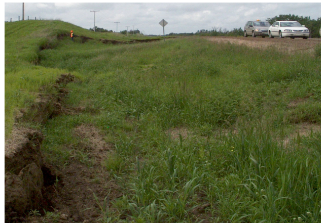
Figure 3. Landslide headscarp in south ditch looking west.
