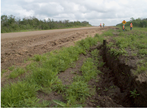
Figure 4. Landslide headscarp in south ditch disrupting ditch drainage with a ditch level higher than the road.
