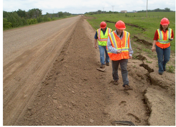
Figure 5. Cracking of the highway shoulder near the west limit of failure.
