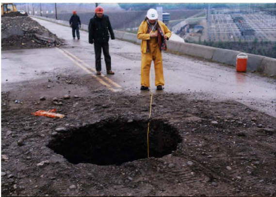
Figure 7: Sinkhole No. 1 at WAC Bennett Dam (1996)
