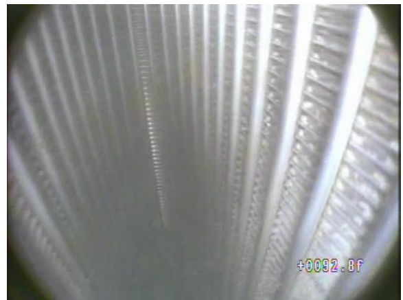
Figure 3F. 28.3 m looking sideways near the narrowest section of the collapsed screen. Distortion of the screen's shape is obvious.
