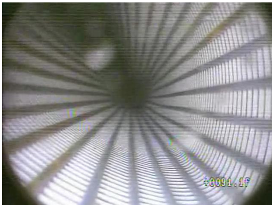
Figure 5C. 27.8 m looking down through the area that had been constricted by the horizontal collapse.
