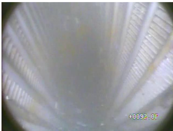
Figure 3C. 28.0 m looking down. The horizontal screen collapse can be seen with the left and right sides pinching in toward the middle.
