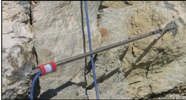
Figure 3. Crack meter (shown before installation was completed).
