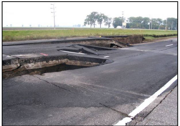
Figure 16. Minnesota site after a major slide.
