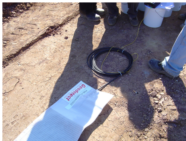
Figure 11. The TenCate GeoDetect® textile fiber optics sensor
