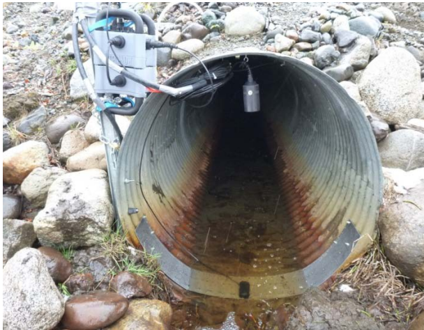
Figure 4 : Flow measurement system in the second year. Water velocity was measured by the lower sensor, shown submerged, and water height by the upper sensor.
