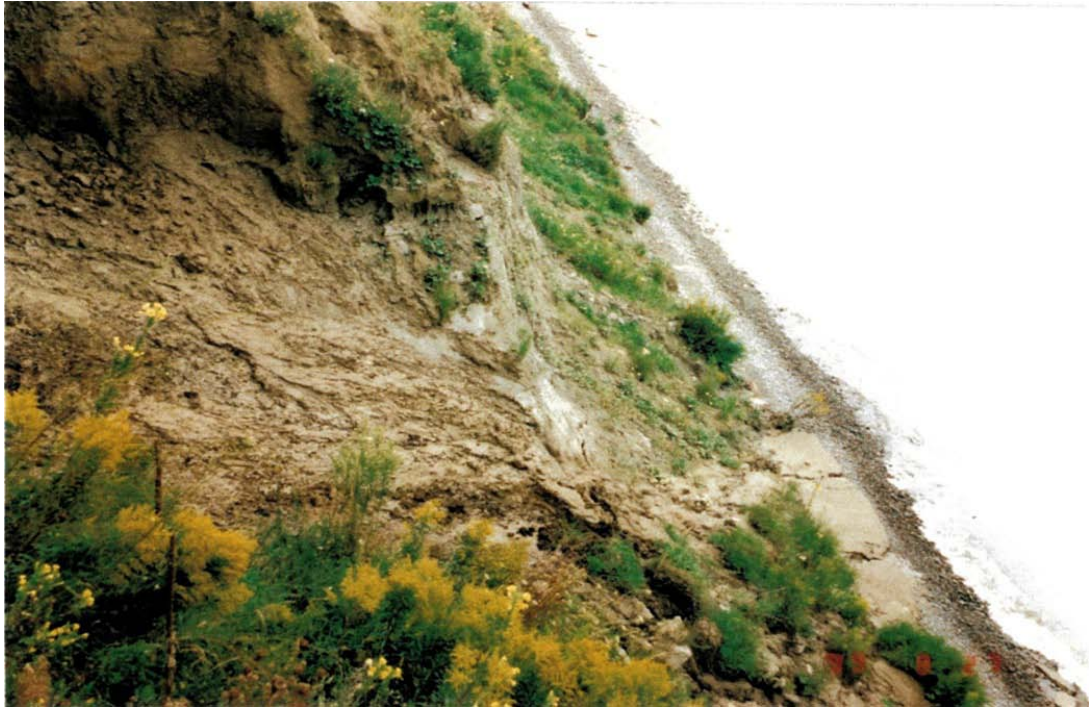
Figure 3. Seepage at Base of Silt/Sand Stratum
