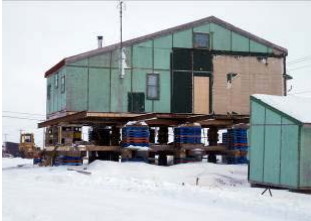
Figure 1. Infrastructure in Baker Lake, Nunavut that has foundational concerns
