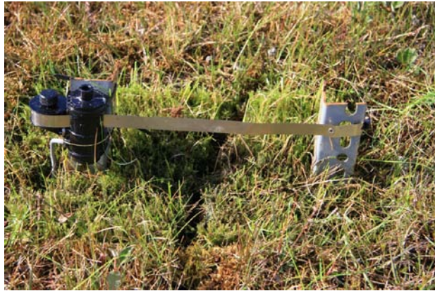
Figure 3 An extensometer installed across a crack.
