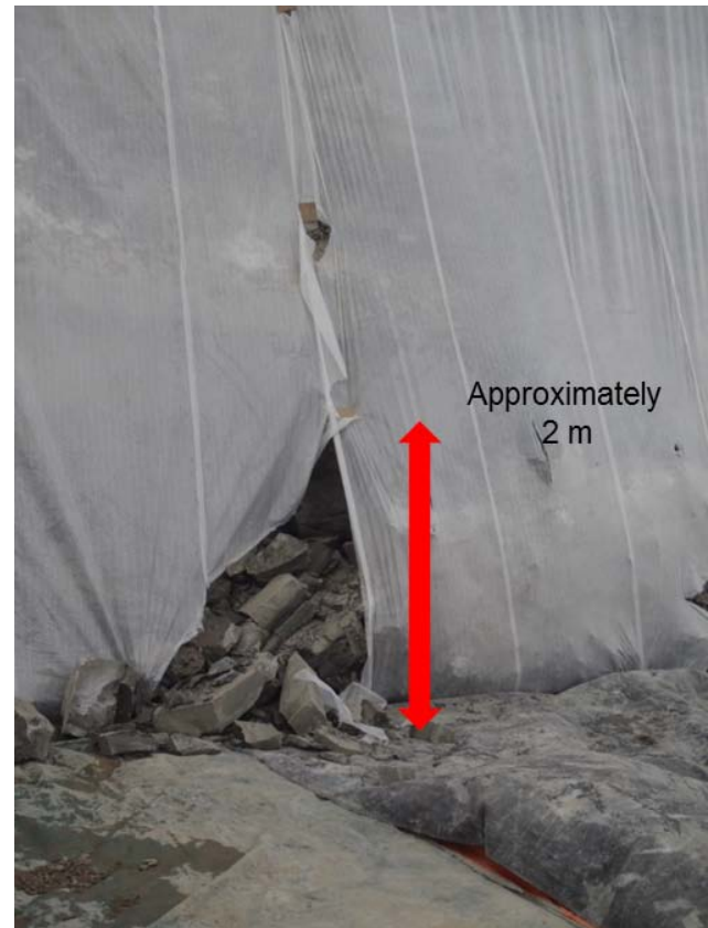
Figure 2: Rockfall Incident Photograph
