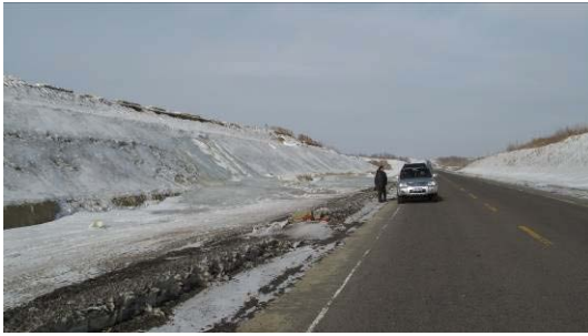
Figure 4. Aufeis on the cutting slope (2010.03)
