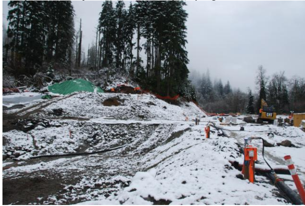
Photograph 3. Perimeter dewatering wells.
