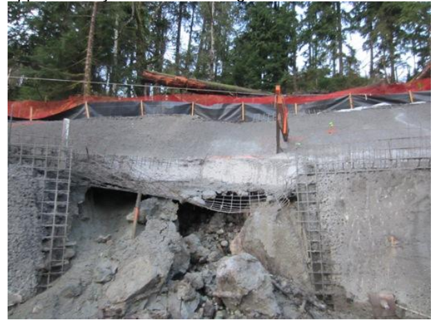
Photograph 4. Collapse of shotcrete facing due to erosion from surface/subsurface flow.
