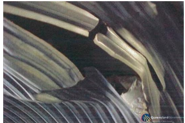
Figure 2. Damage to a CSP culvert due to corrosion (DTMR, 2013).
