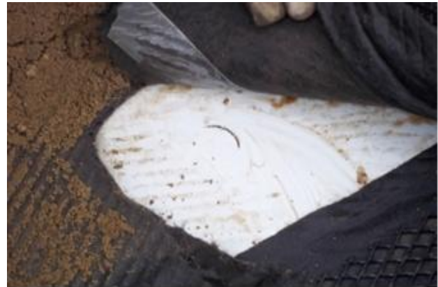
Figure 4. Detected damage on partially exhumed geomembrane (Ramsey et.al., 2012)
