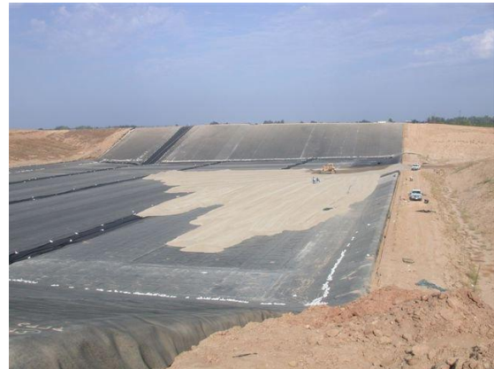
Figure 2. Poor cover soil placement (note the lack of a distribution pattern) without CQA.
